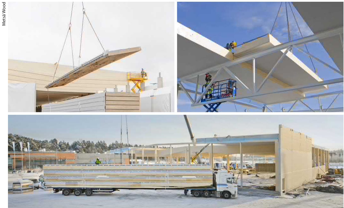
Figure 2.40. Installation of roof elements with LVL purlins. Metsä Fibre pulp terminal, Vuosaari, Helsinki, Finland; Karisma, Lahti, Finland; Skanssi, Turku, Finland.
