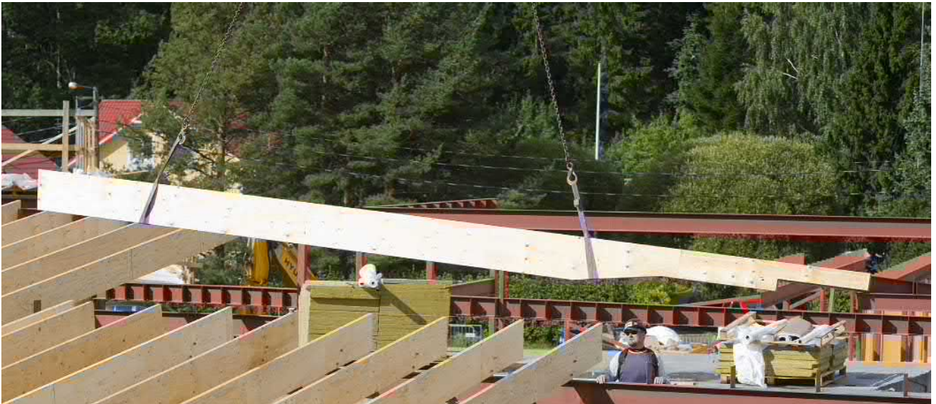
Figure 2.31. Notched rafter end at the front roof overhang.
