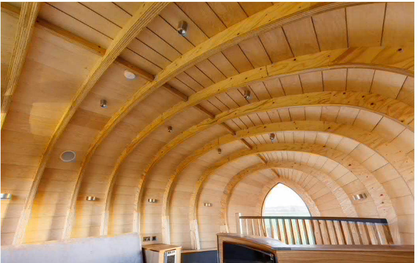
Figure 2.91. LVL-C arches for the roof structure of a windmill, UK. The structure consists of several curved members.
