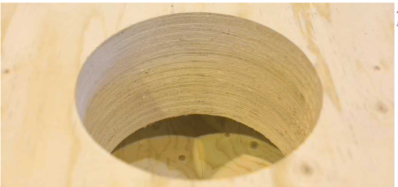
Figure 1.50. Hole in an LVL beam.
